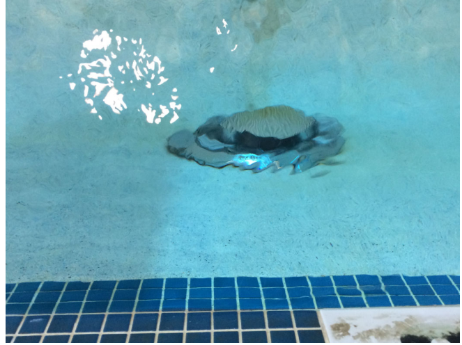
Broken pool light
