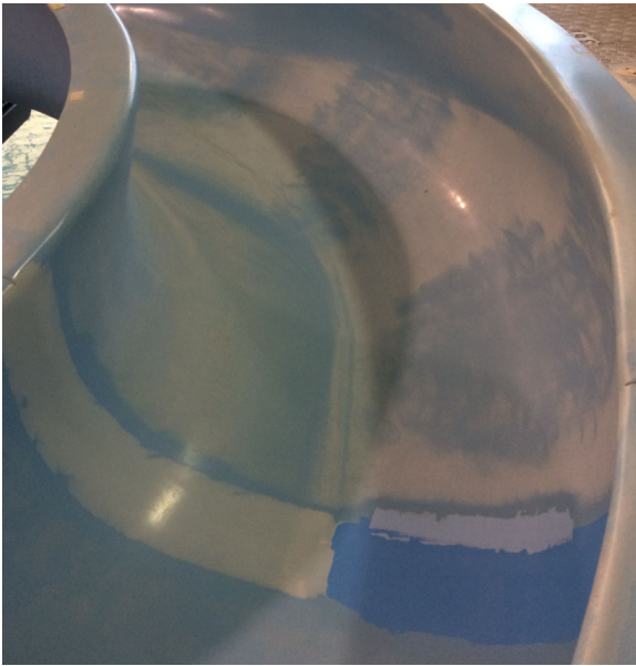
Worn slide with cracked seams
