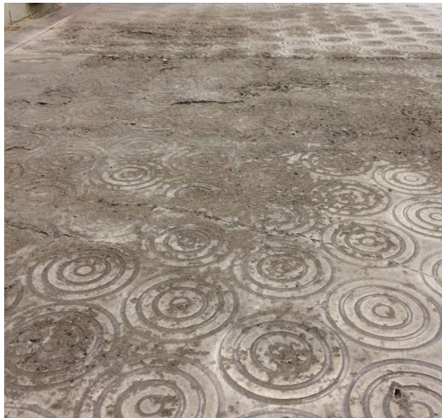
Deteriorated pool deck
