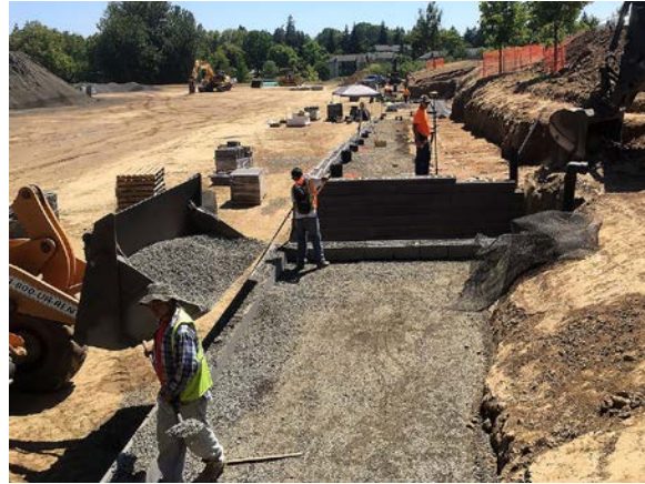
Workers for Benchmark Contracting build a retaining wall as part of the project to create a new synthetic turf athletic field at Conestoga Middle School.
