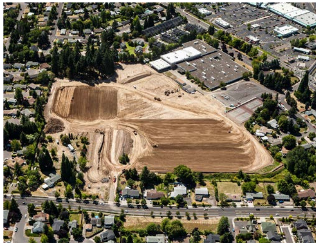
Initial work on the new community park in Aloha has included preparing the soil for side-by-side athletic fields. Grading is scheduled to be complete by fall. © Oregon Aerial Photography
